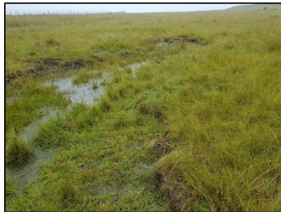
b) Head-cut erosion of Seasonal Seepage Wetland downstream of existing, closed landfill.
