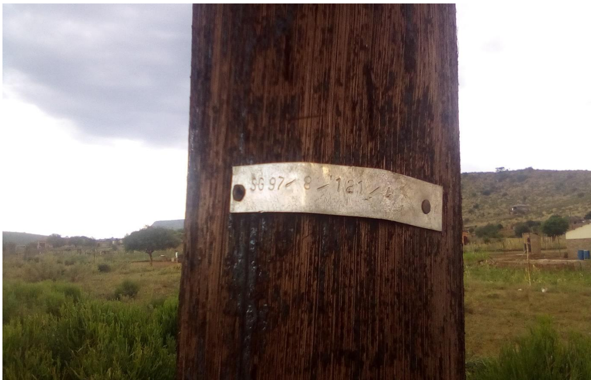
Pole number of the existing line
