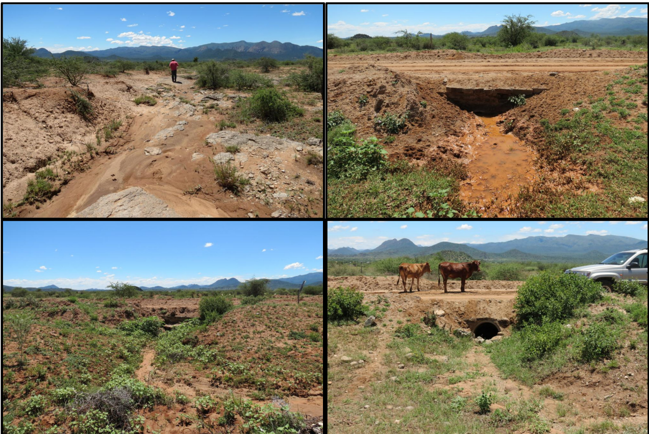
Figure 6: Drainage channels and storm water pipes
