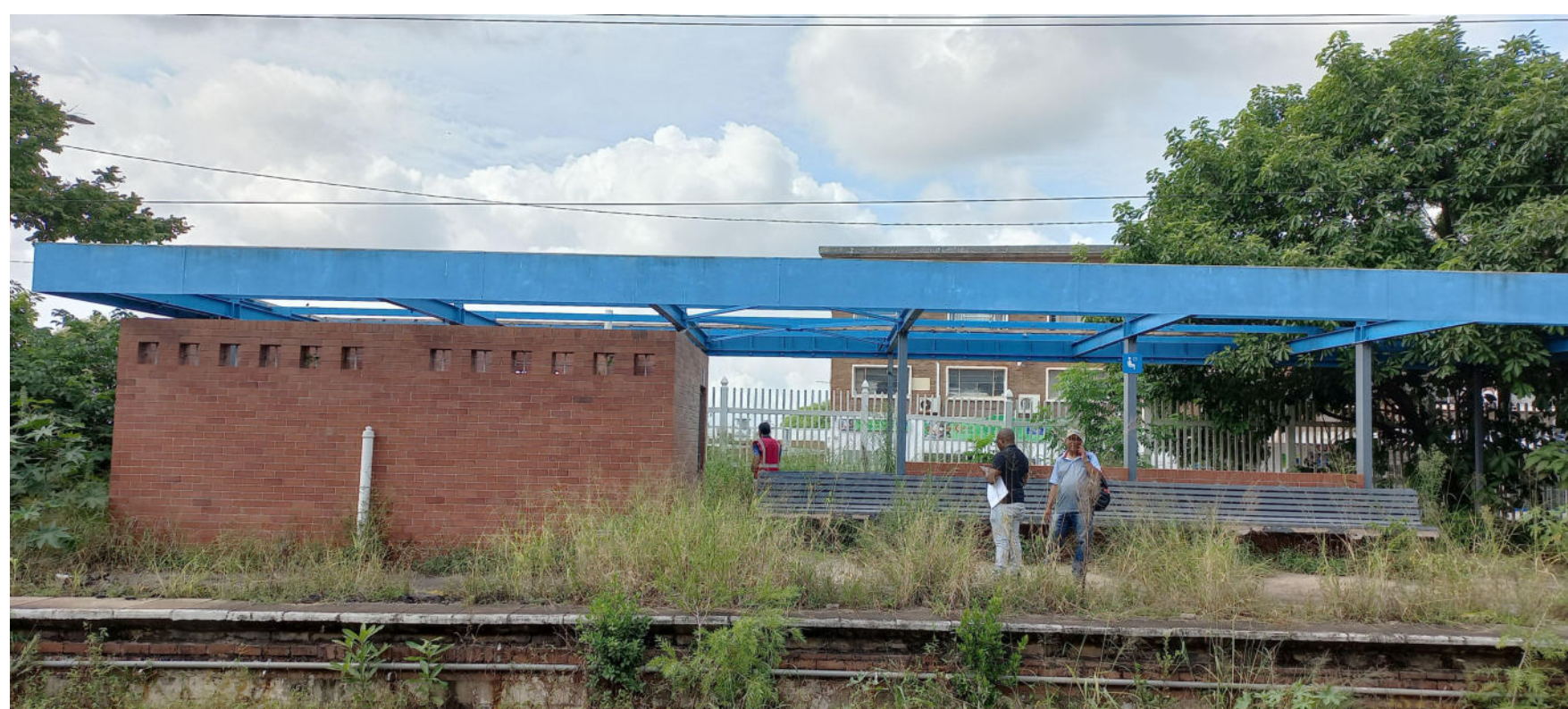
7. EXISTING PUBLIC ABLUTION & COVERED SEATING AREA (UNLAWFUL WORK)
