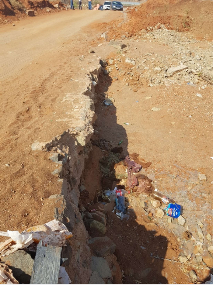
Figure 6: Downstream from the crossing showing the dry stream bed and undercut slab of the current infrastructure
