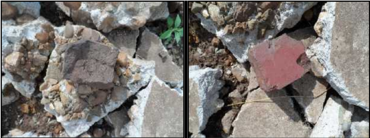
Figure 30 - Remains of house foundation - the bricks have been salvaged.
