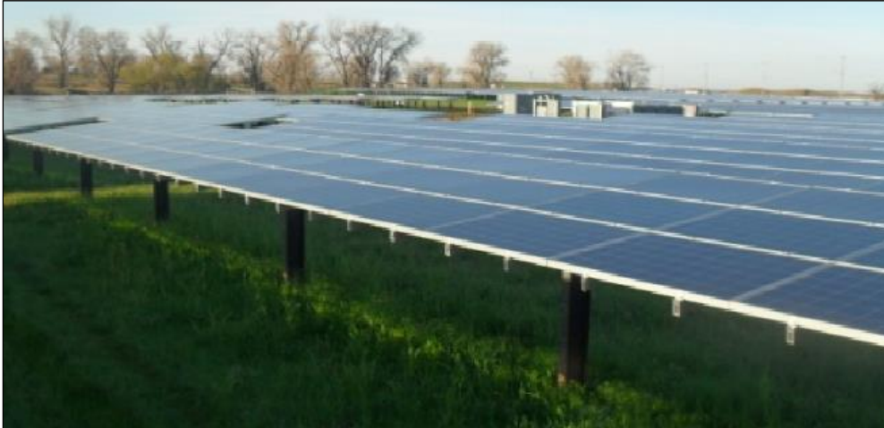
Figure 6: Frontal views of the PV arrays mounted on 1-axis horizontal tracker
