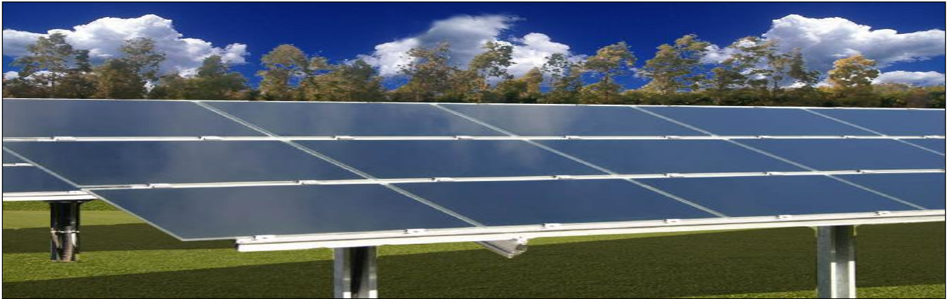
Figure 4: Frontal view of PV arrays mounted on fixed mounting systems
