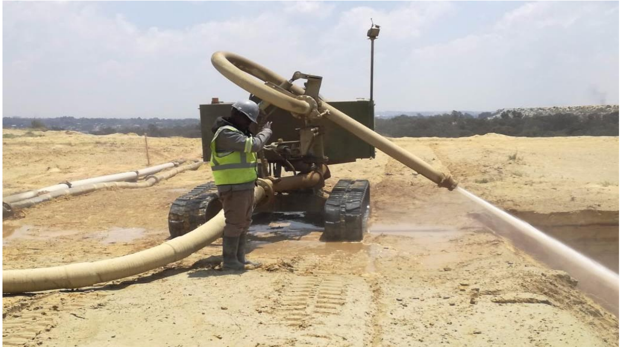
Figure 2-2: Mobile tracked hydraulic monitor on a tailings facility in South Africa
