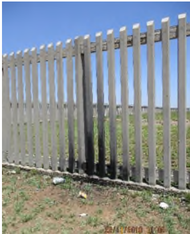
Burning and litter along the fencelines
