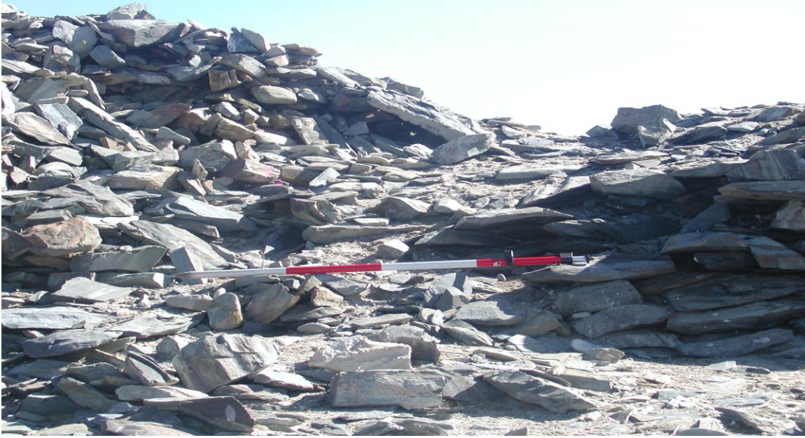
Collapse between façades 2d and 2e.
