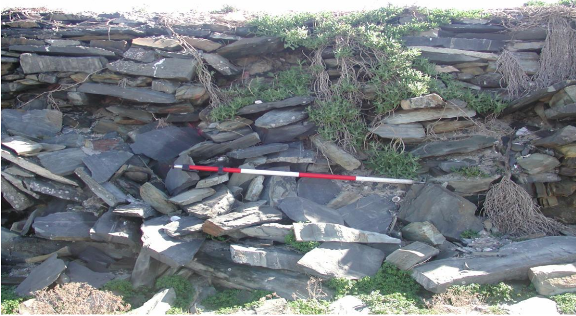
Collapse between façade 2a and 2b.
