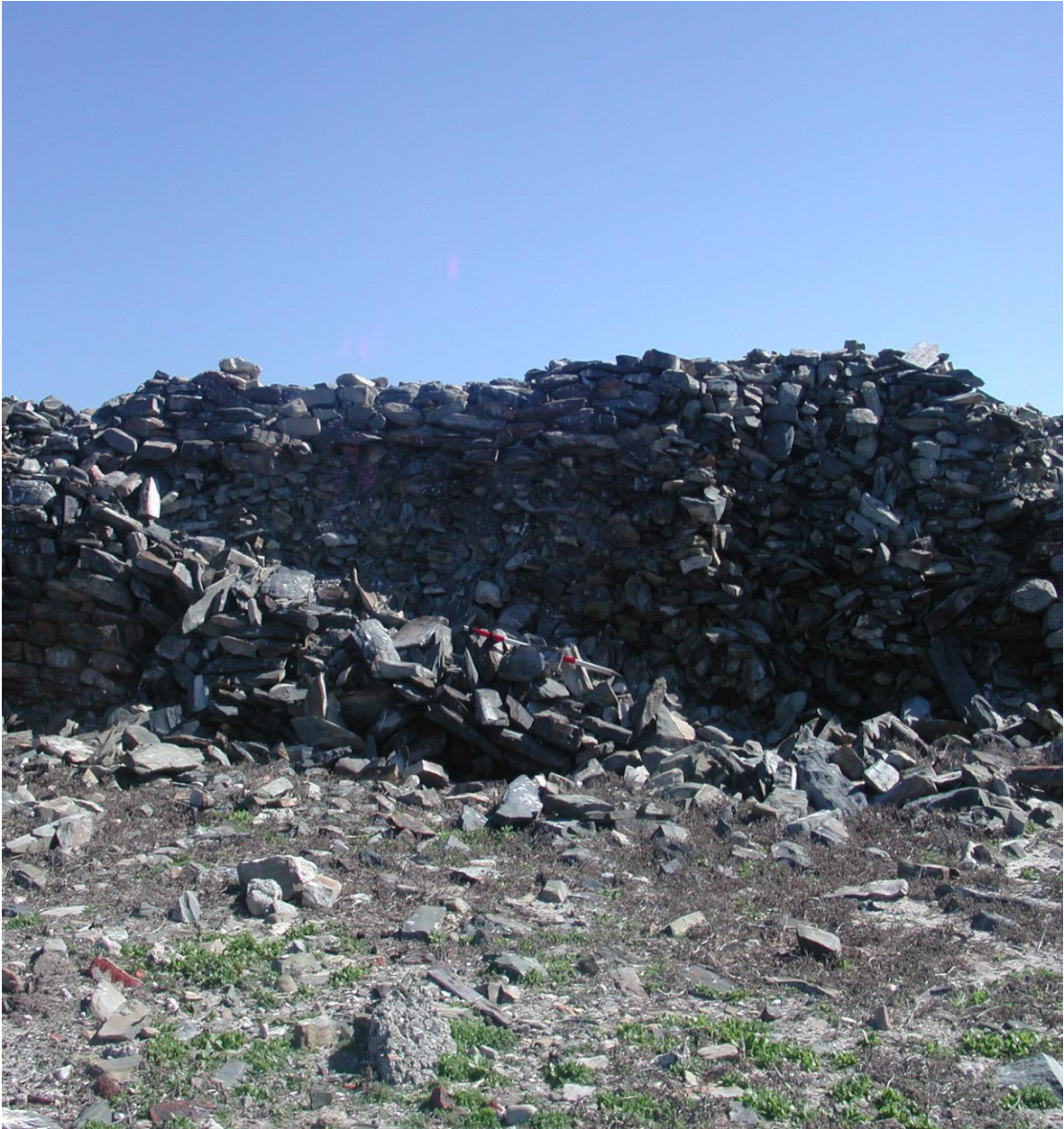
Collapse between façade 2e and 2f
