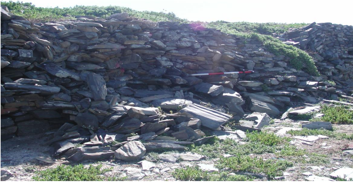
Collapse between facade 2b and 2c.
