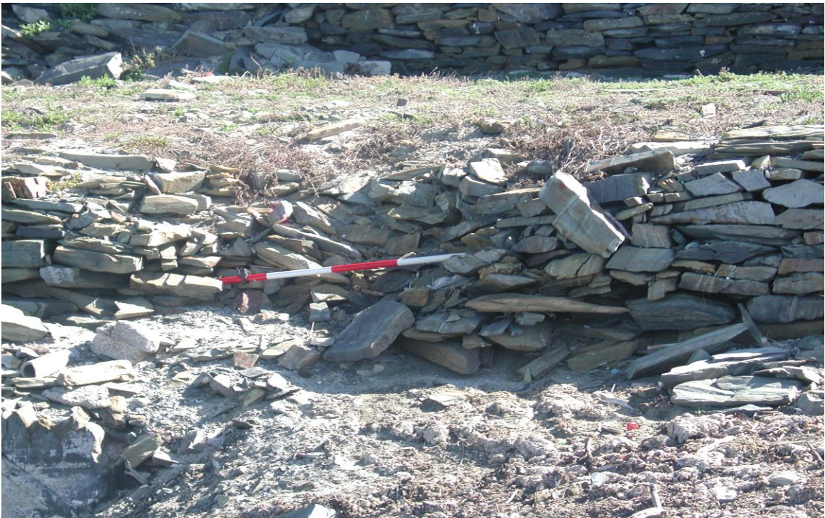
A 1.5 m long collapse separates façade 6b from 6c.
