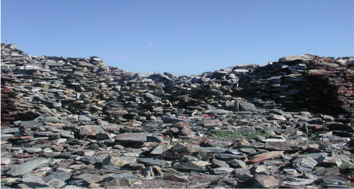
A 6m long collapse separates façade 2g from 2h.
