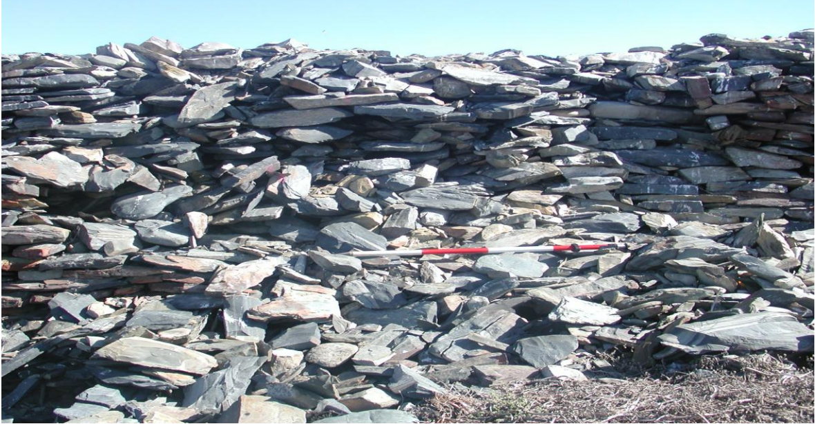
A 2m long collapse of the top blocks separates façade 2f from 2g.
