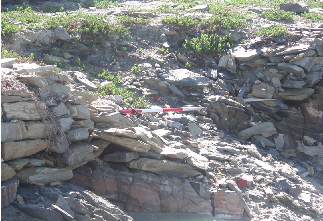
A 2.5m long collapse separates façade 6d from 6e.
