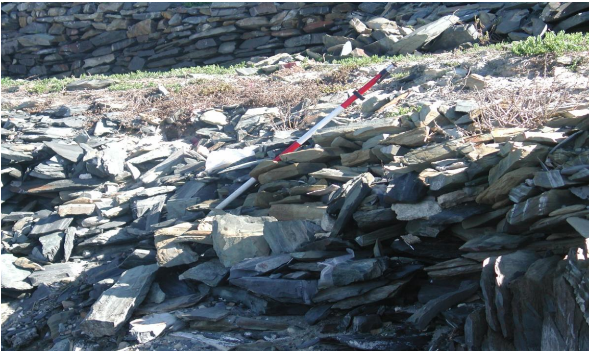
A 3m long collapse separates façade 6c and 6d.
