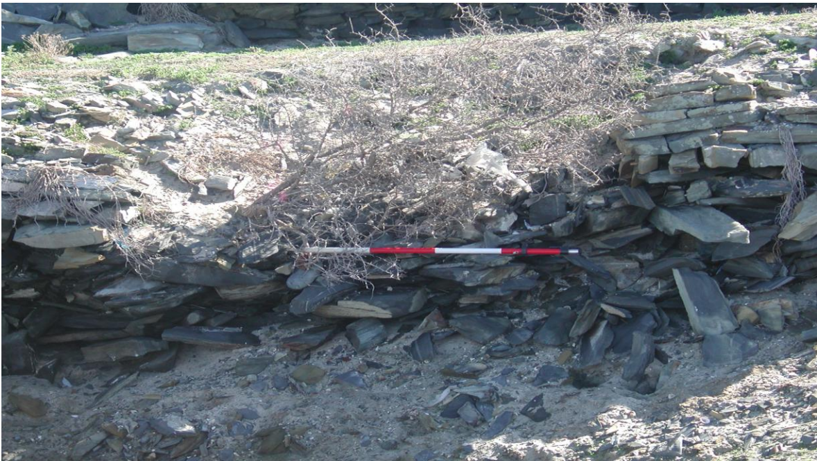
A 2.5m long collapse separates façade 6a from 6b.
