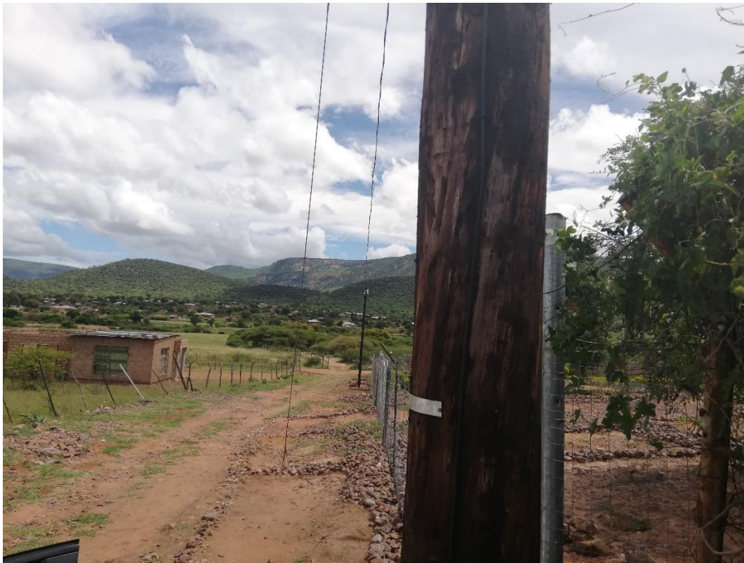
Figure 1 T- off point from existing MV power line
