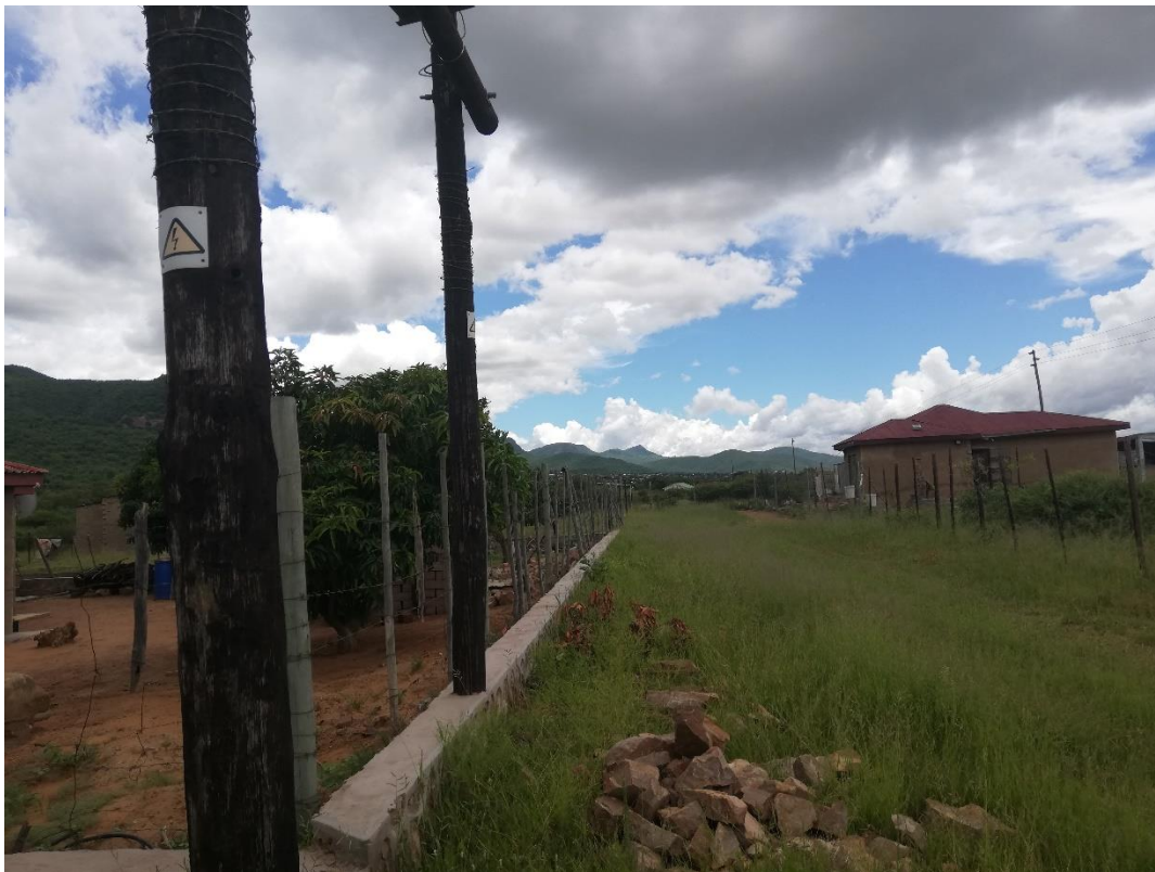
Figure 6 Transformer t-off point
