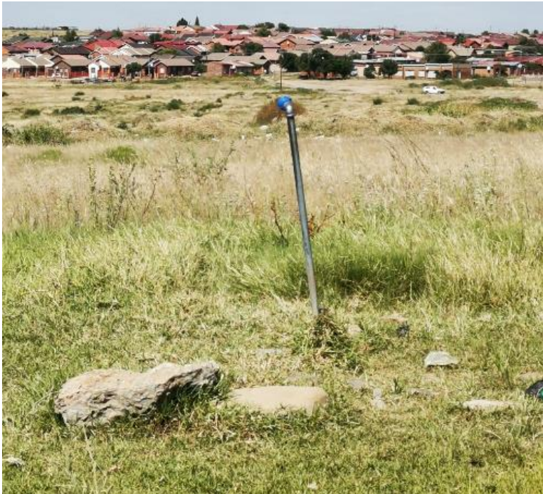
Figure 16 Capped water standpipe on existing pipeline
