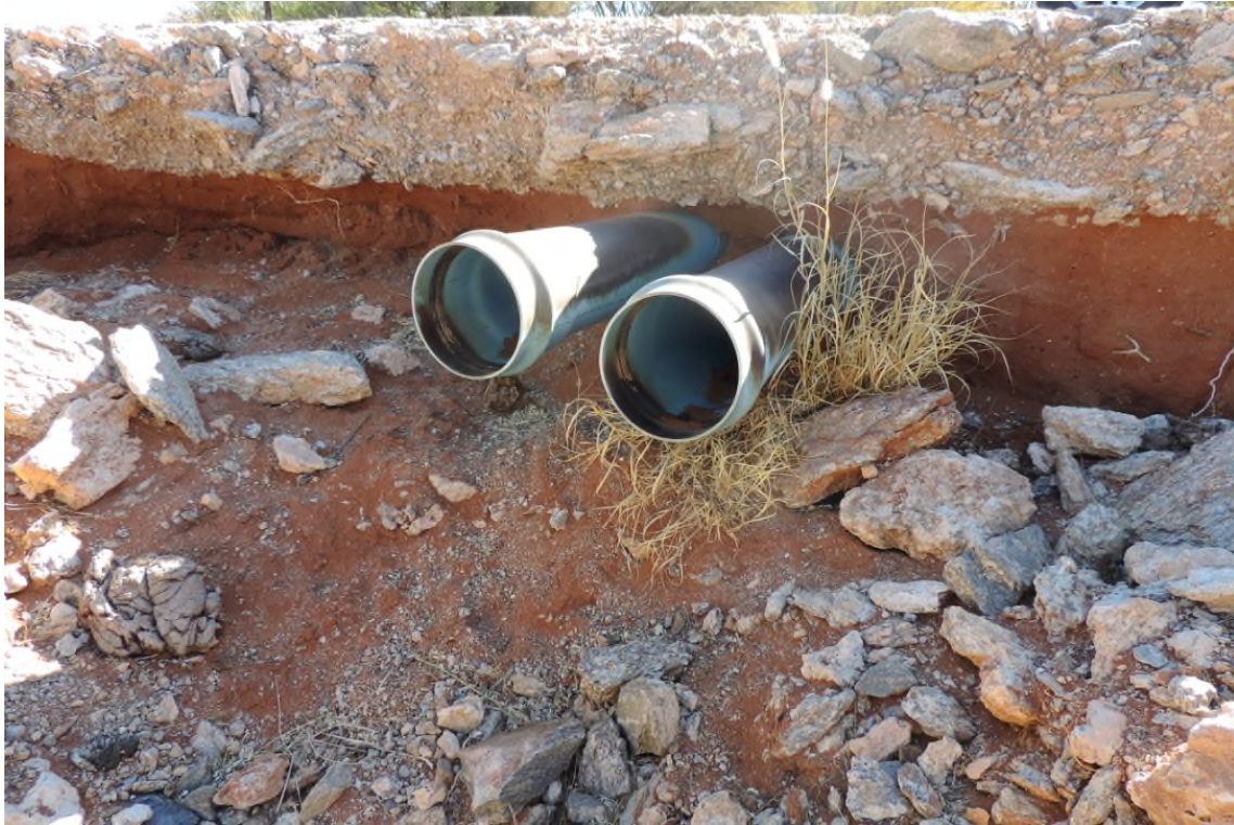
Figure 6 Hardpan carbonate material (underlying the Coega soil form) has been used to stabilise the sandy red apedal soil where farm roads crossed over preferential flow paths
