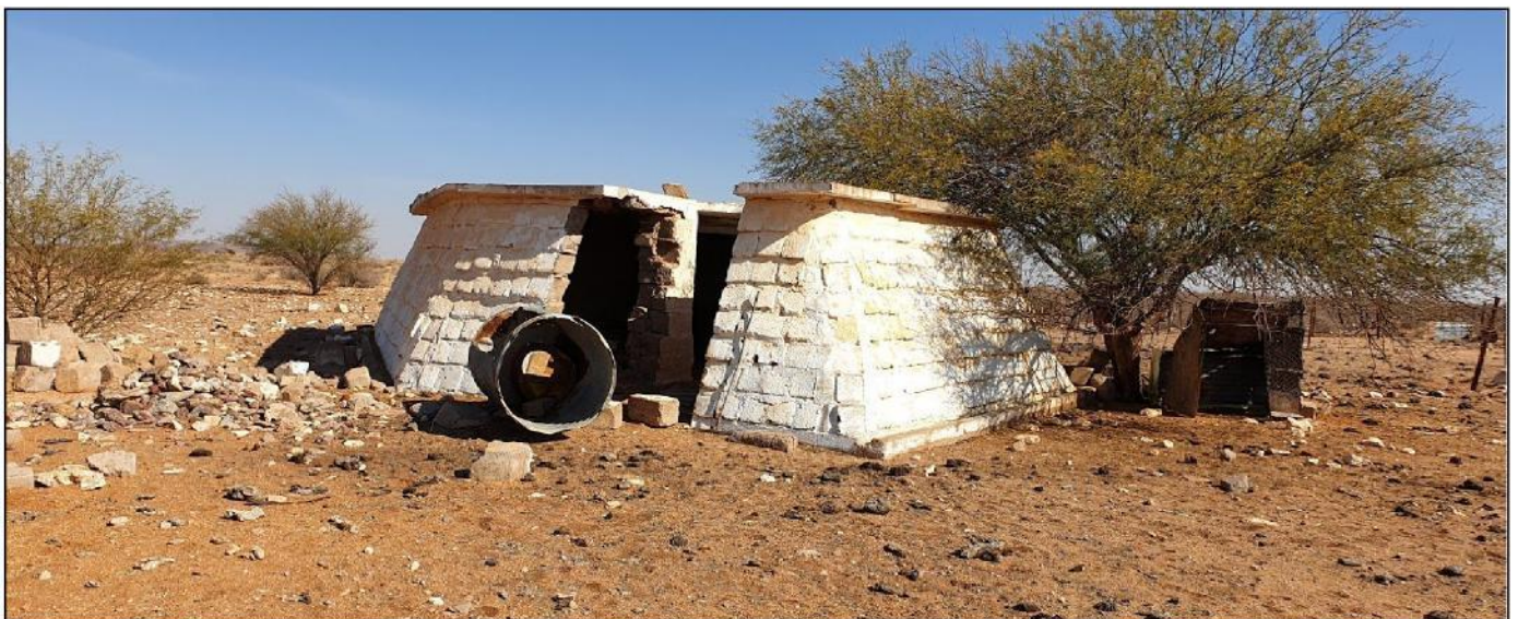
Figure 6.4 Remnants of bunker used for storage of explosives used during mining of tungsten (Pt 22)
