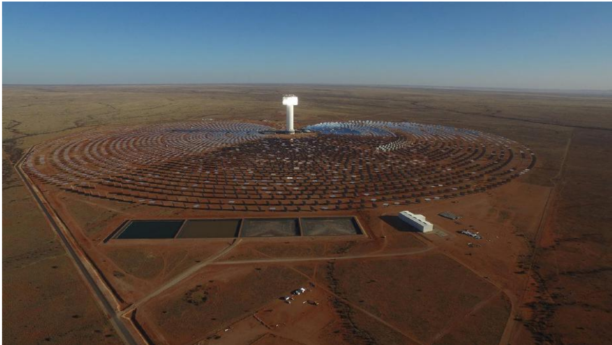
Figure 4.3: Operational Khi Solar One located in the southern corner of Portion 3 of the Farm McTaggarts Camp No. 453 (source: www.energy.org.za )
