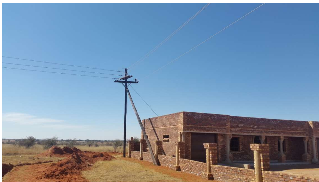
Photo 17: SG line pole No 91 going to Ipelegeng Extensions 8 and 9
