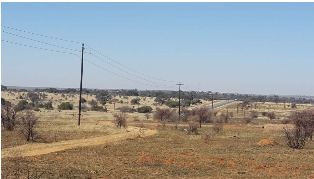
Photo 16: Eskom Line SG – along Vryburg road
