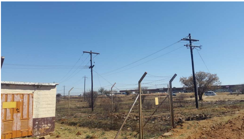
Photo 13: Start of line at Swartz Street MLM Substation
