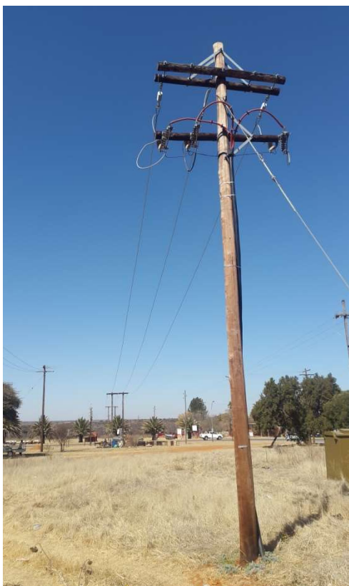
Photo 15: View of 11kV (mink) overhead line from the Eskom Schweizer Reneke Munic 88/11kV Substation
