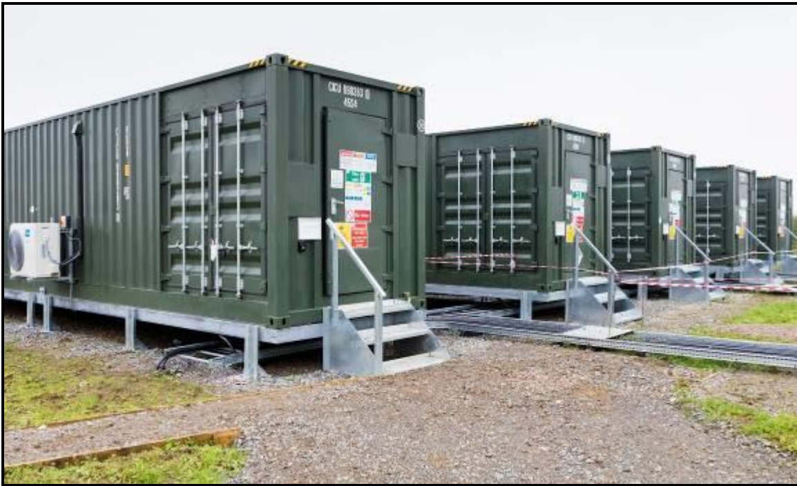
Photograph 1.1: Example of BESS located in storage containers
