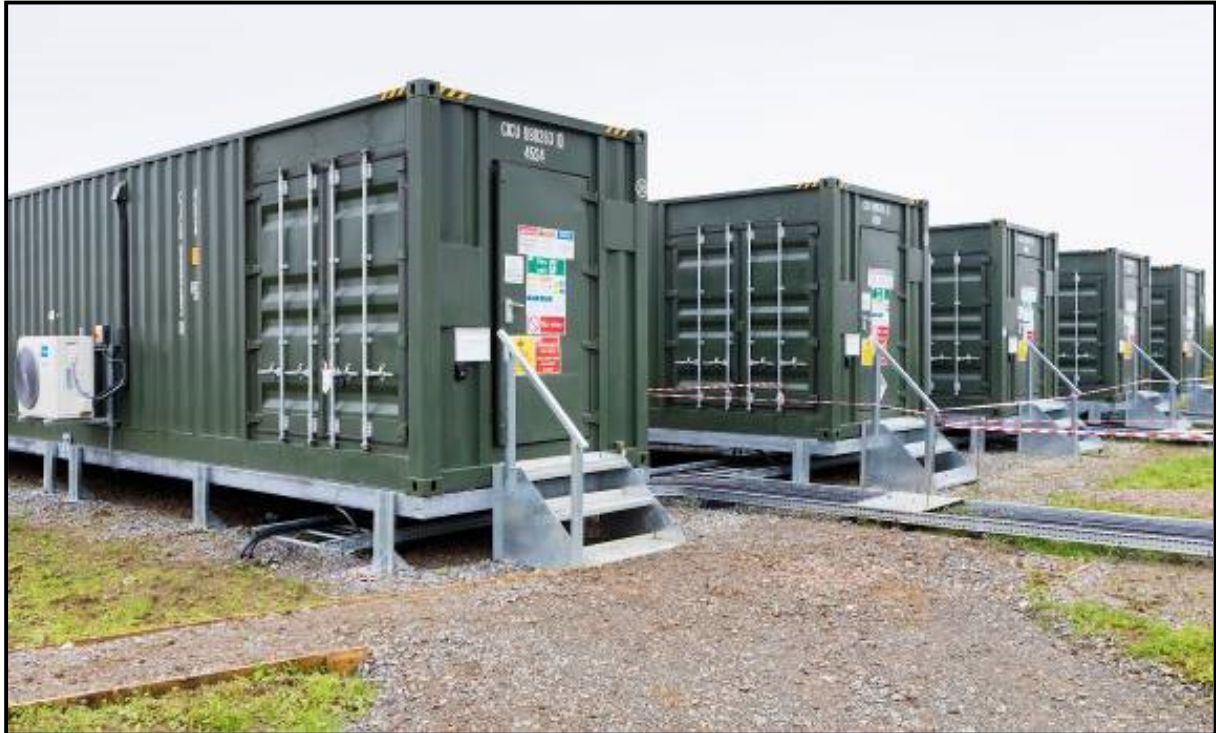
Photograph 1.1: Example of BESS located in storage containers
