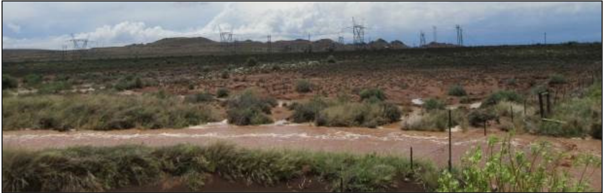
Photograph 3.3: Portion of Gamma substation located just to the north of the R63
