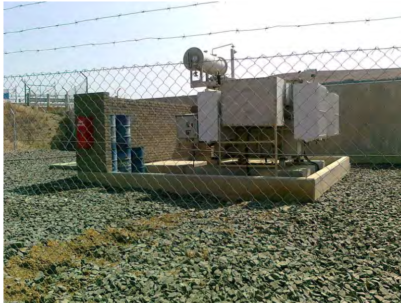
Figure 4 Merino Hydro Power Station Transformer
