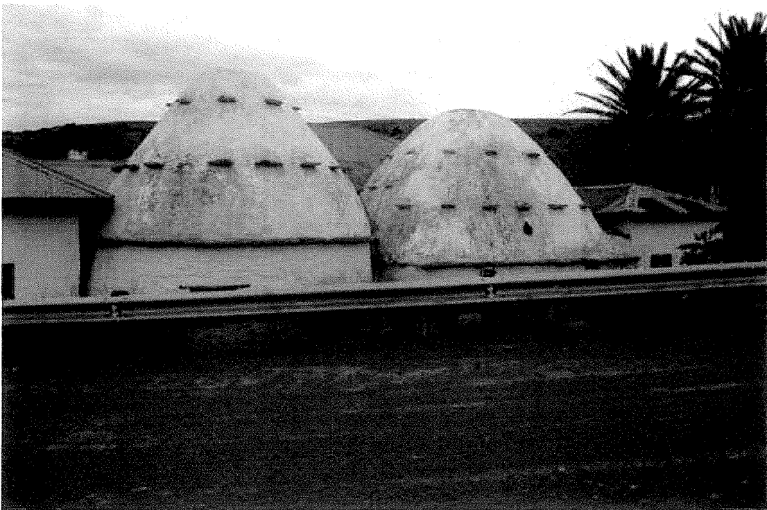
Figure 24. These corbelled dwellings, declared national monuments' are the two most important buildings that may be affected by heavy duty transport vehicle. The main road literally passes within four meters of the stone constructions.
