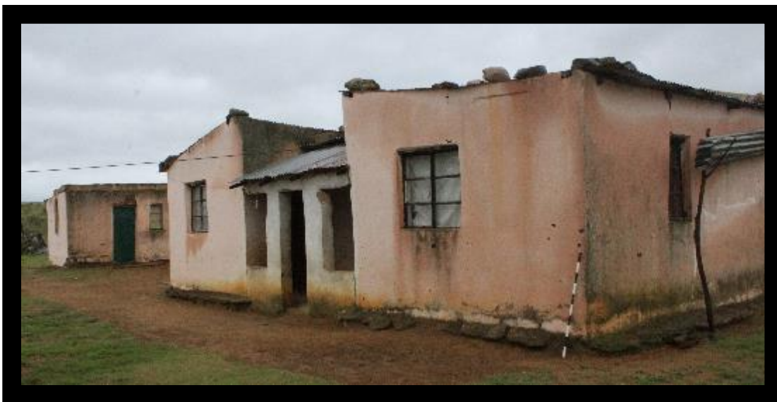
Figure 9.18: Example of house in poor condition.
