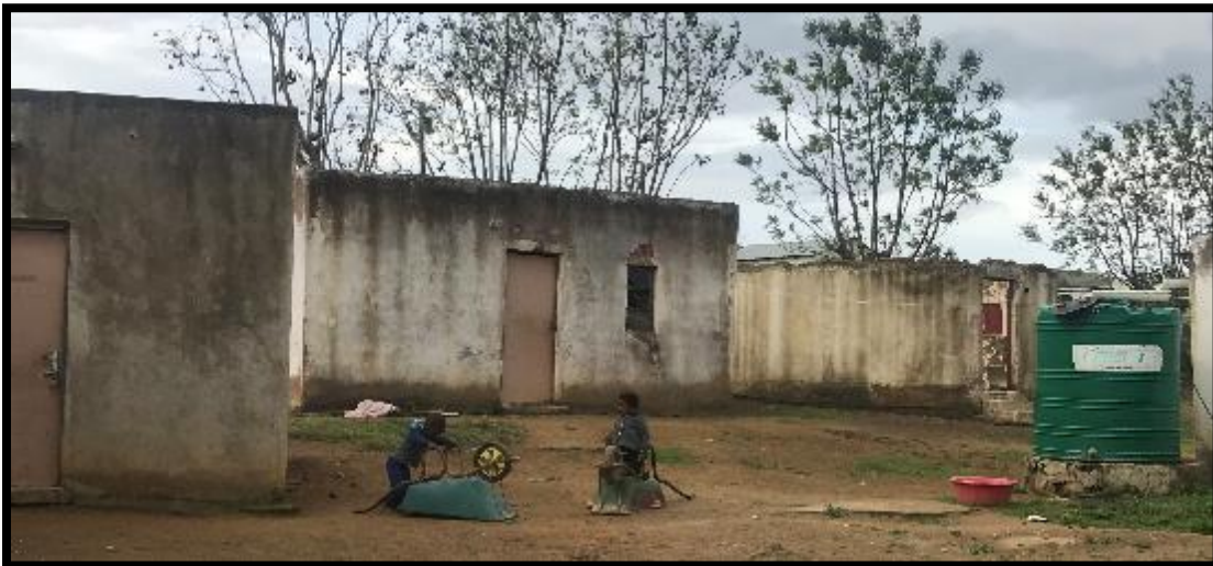
Figure 9.20: Example of house in poor condition
