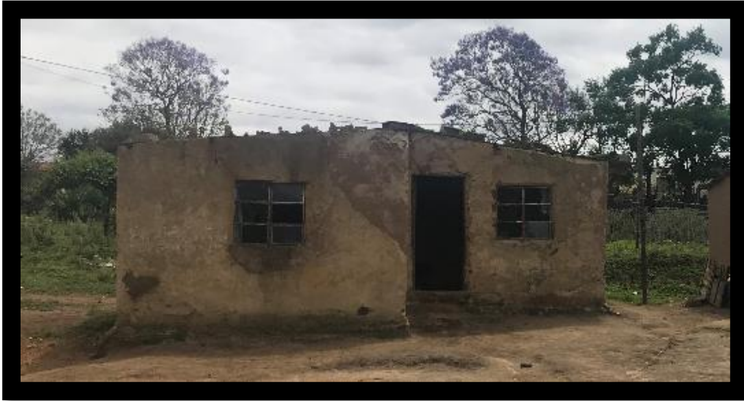
Figure 9.17: Example of house in poor condition.
