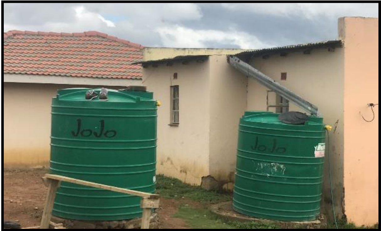
Figure 9.23: Jojo tanks used to store water
