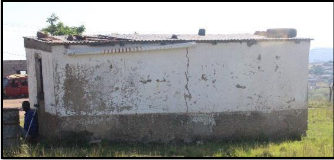
Figure 9.19: Example of house in poor condition.
