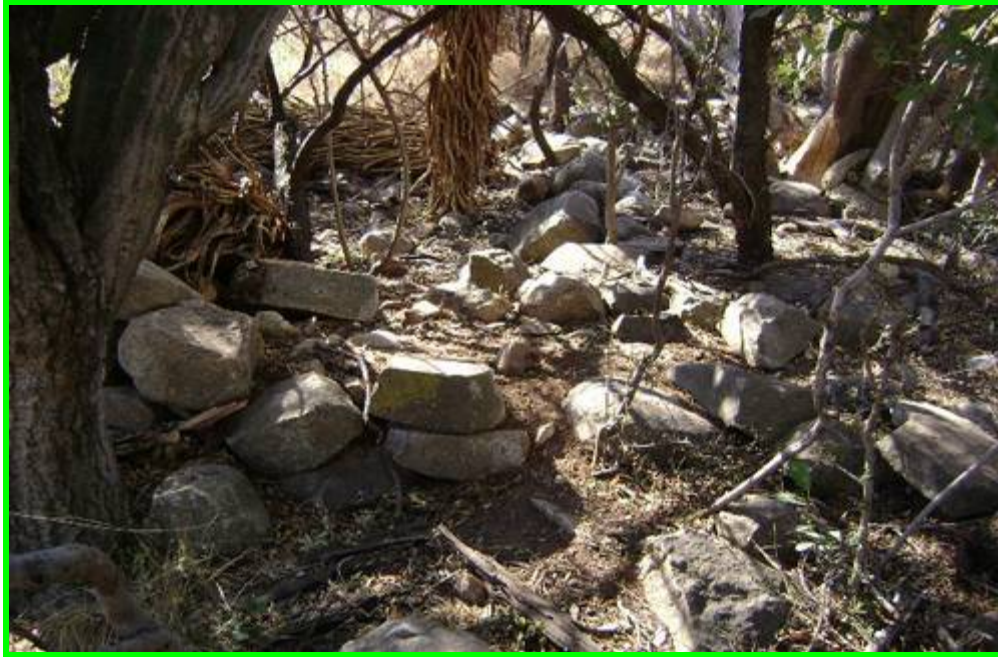
Figure 7: A section of dilapidated stone wall.
