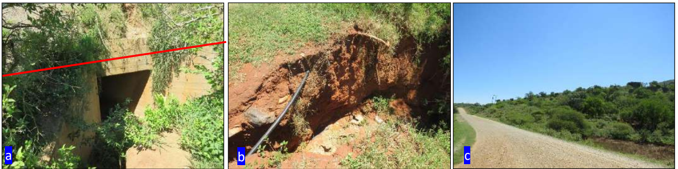
Figure 40: (a): Existing watercourse structure which the proposed pipeline would traverse (red line); (b): Existing pipeline crossing a watercourse. Note erosion associated with the watercourse; (c): A section of the road where the proposed pipeline would run parallel to as well as the associated vegetation.
