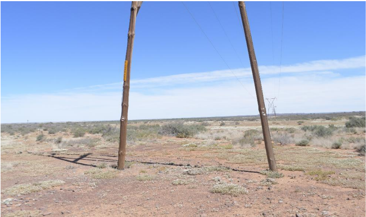
Figure 2: The existing Cuprum - Karoo 1 66kV overhead line which runs just east of the proposed development area.
