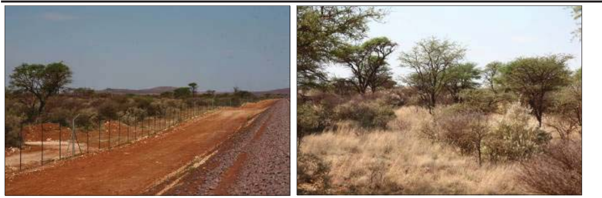
Figure 8 The Sishen loop site, illustrating the dense nature of the intact vegetation at the site, as well as the extent of cleared ground that has been created by construction activities for the new line at the site, being built by Kumba Iron Ore.
