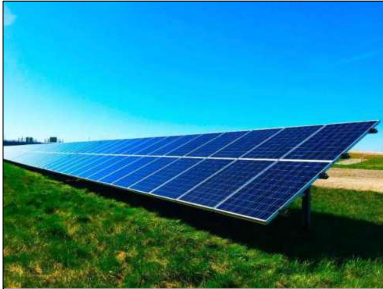
Figure 13 : Tilted Solar Panels with landscaped surface area
