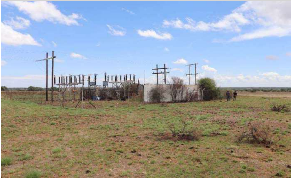
Figure 4: Existing power substation on the property
