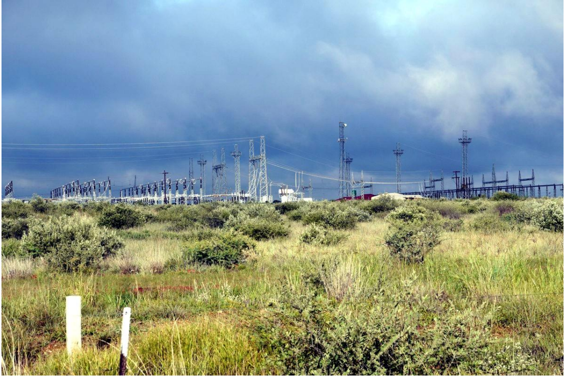
Plate 1, Existing Mookodi 400/132kV Substation.
