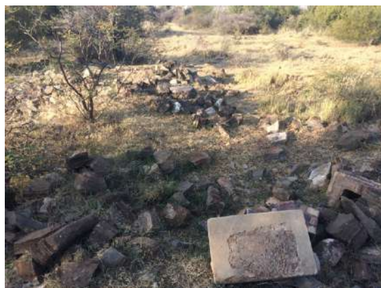
Figure 33 - Collapsed structure at site 023, showing a mix of constructive elements (concrete, bricks and cement).
