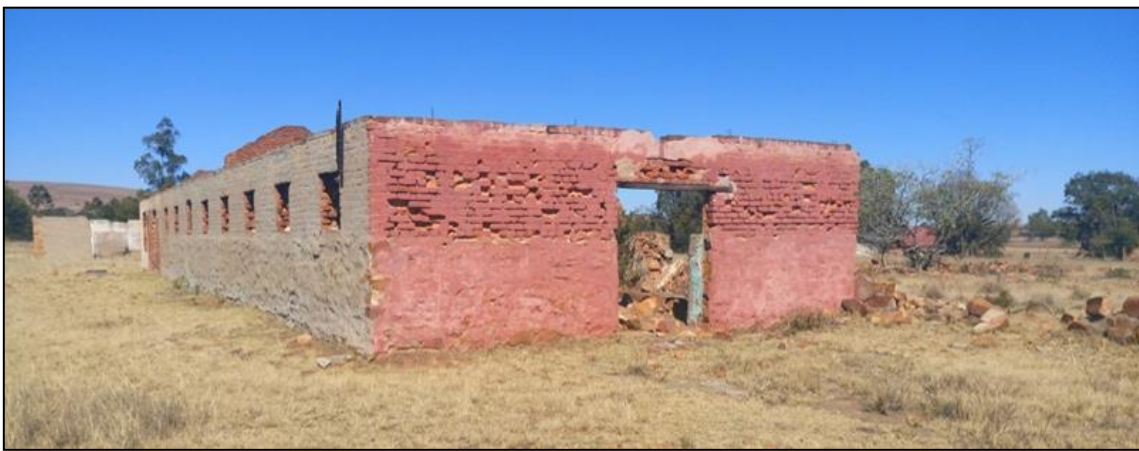
Figure 13: View of the northern wall of the main dairy building showing modern bricks with a concrete lintel above the doorway. The stone and cement kraal is visible to the right.
