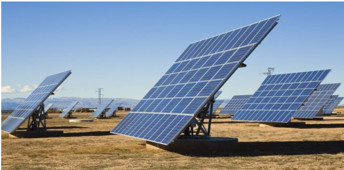
Figure 2: An Example of a photovoltaic array
