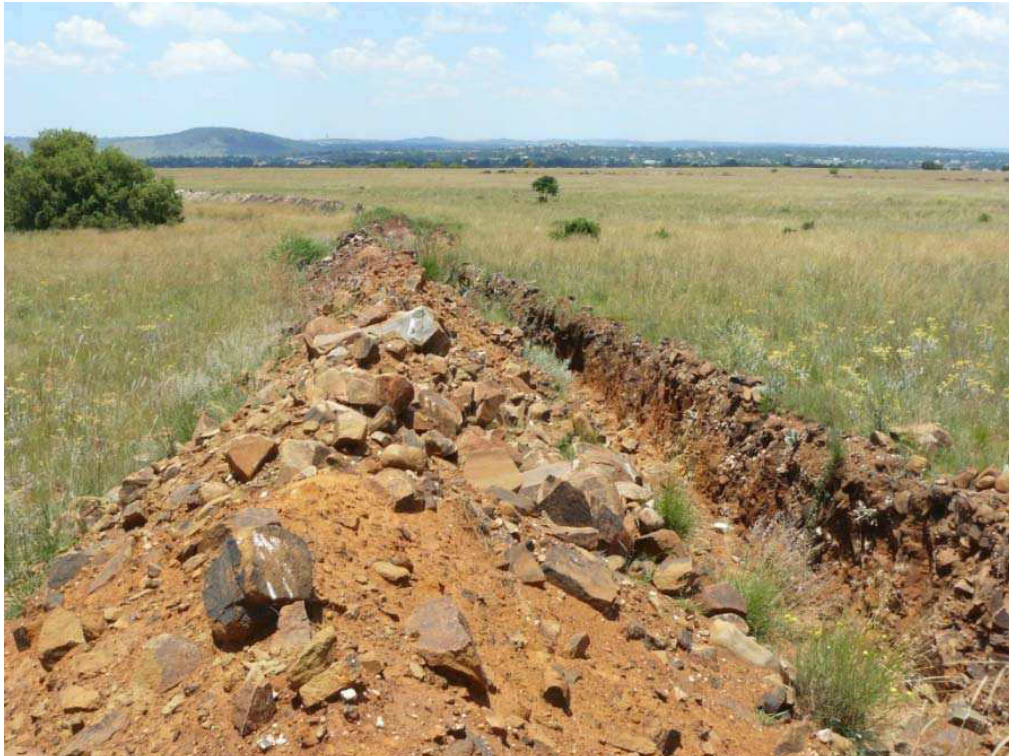
Photo 4: Services trench dug through part of the Rocky outcrop vegetation along the eastern boundary of the site
