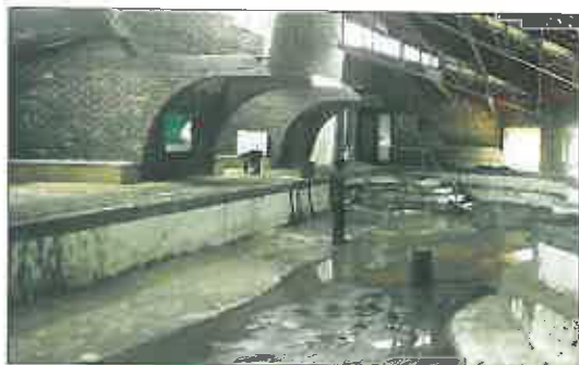
The undercover swimming pool, after being damaged, heavily damaged. Photo: Justin Steyn
