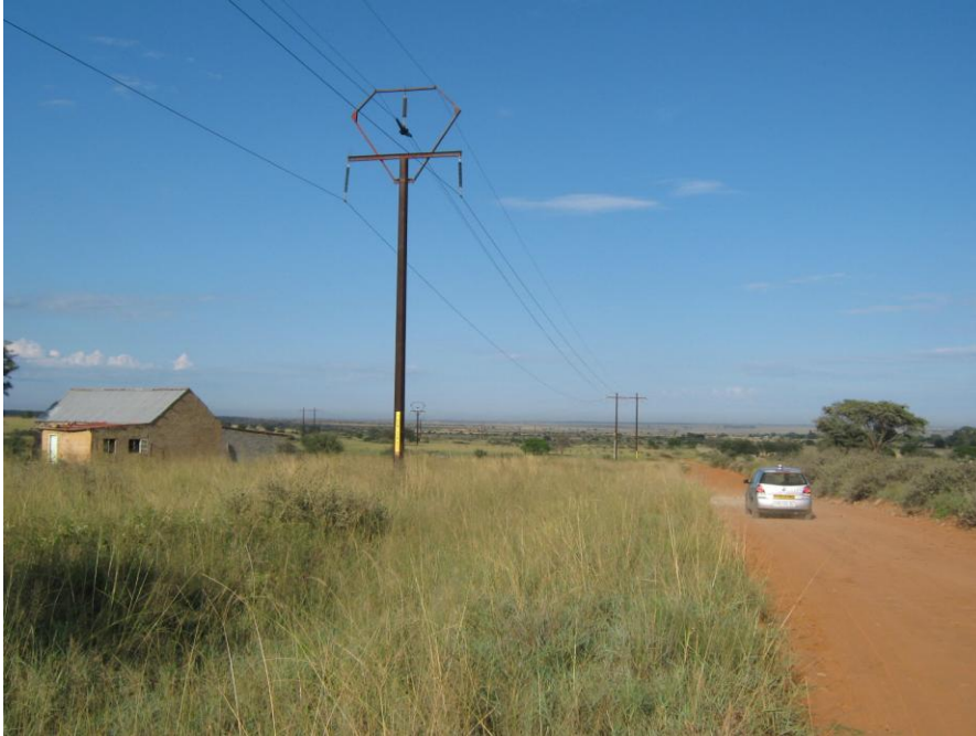
Figure 12: Existing power lines and farm house along a portion of the proposed Bophirima Substation to Kalplats Substation route
