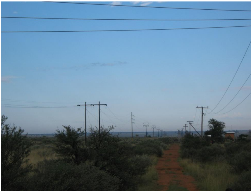
Figure 35: Existing power lines near the Bophirima substation
