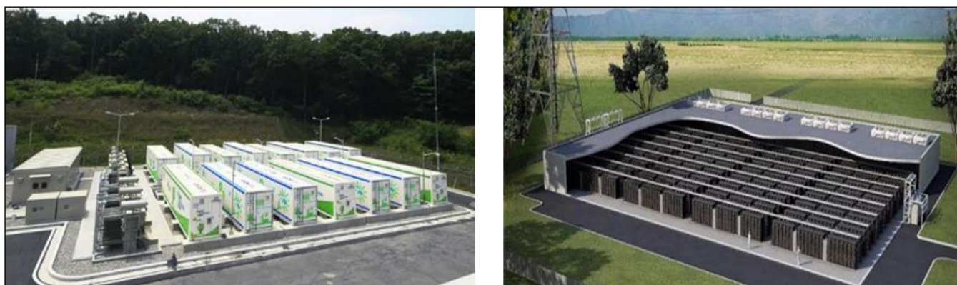
Figure 5. Battery Energy Storage System (BESS)
