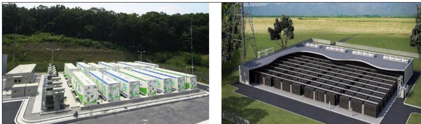
Figure 5. Battery Energy Storage System (BESS)
