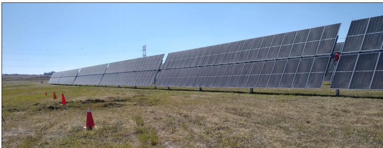
Figure 4. Front views of the PV arrays mounted on horizontal 1-axis tracker
