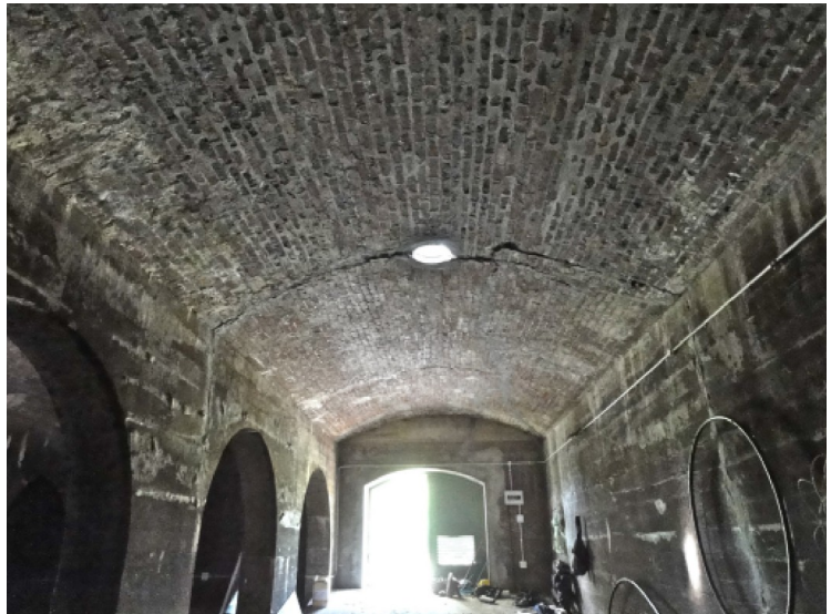
Cistern: view of interior. Note structural crack running through the vault at mid-span, through piers and perimeter wall.
