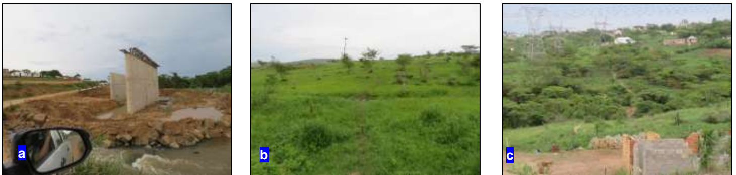
Figure 23: (a) View of the construction status of the new structure along the Mpolweni River; (b) A watercourse crossing point following an existing footpath within the southern portion of the Mpolweni project area; (c) A watercourse crossing point following an existing footpath within the western portion of the Mpolweni project area.
