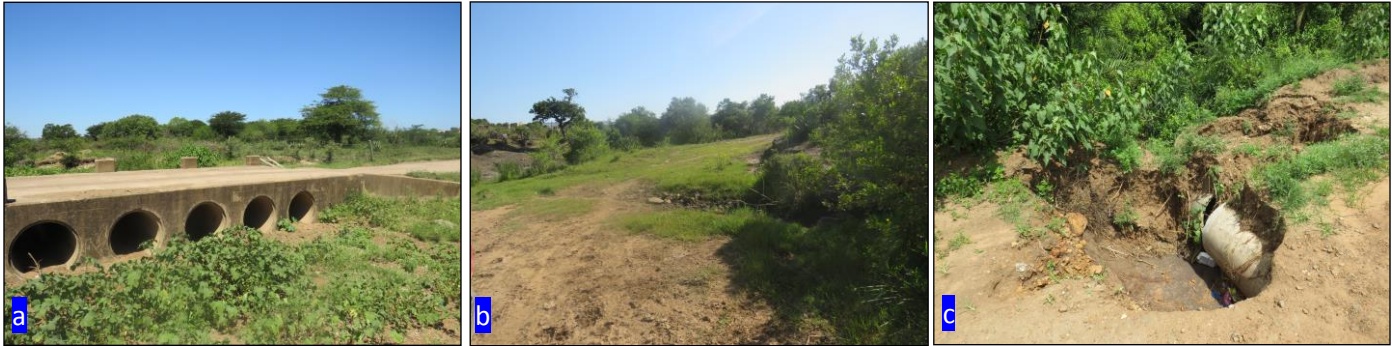
Figure 12: (a): Large culvert that crosses the watercourse where the water pipeline will cross at WC27. (b): Road crossing a watercourse at the same location as the pipe crossing WC43; (c): Heavy rains have caused the old culverts to start eroding.
