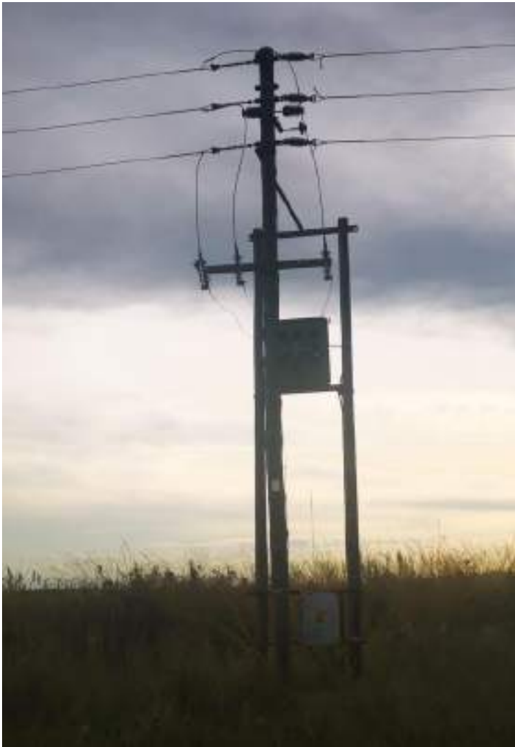
Figure 21 Existing electricity supply line
