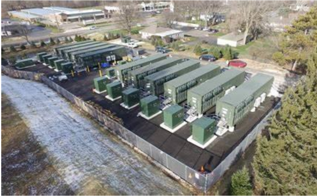
Plate 2 - Typical Battery Energy Storage System
