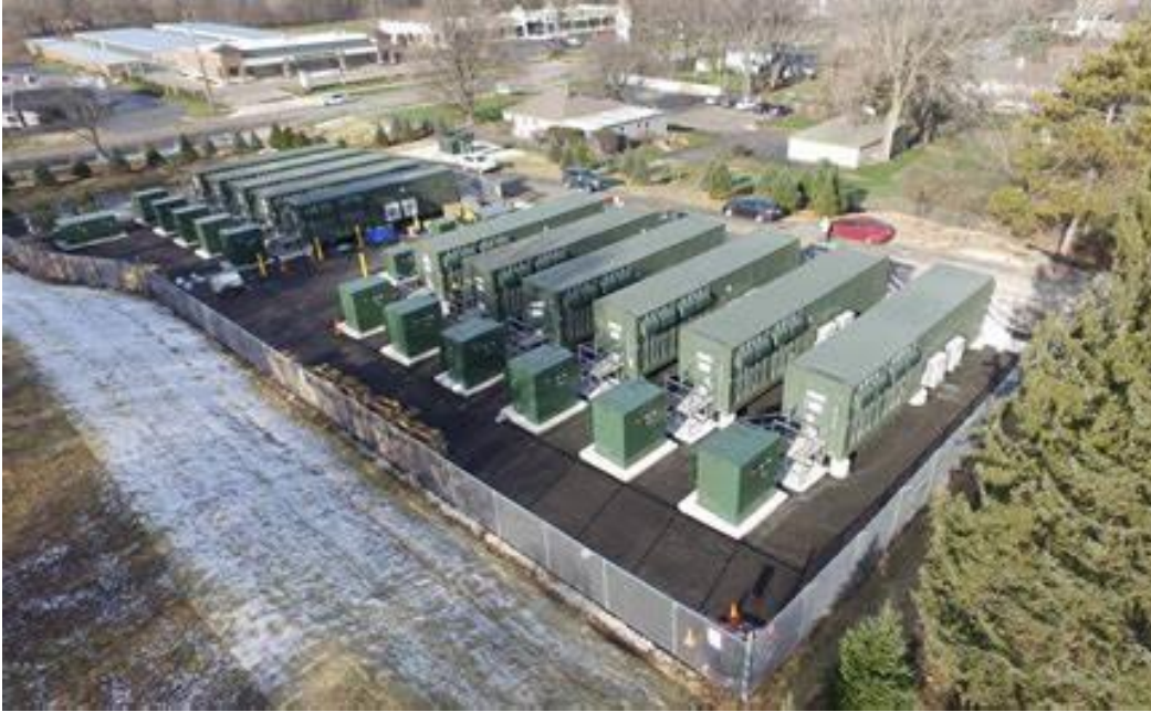
Plate 2 - Typical Battery Energy Storage System
