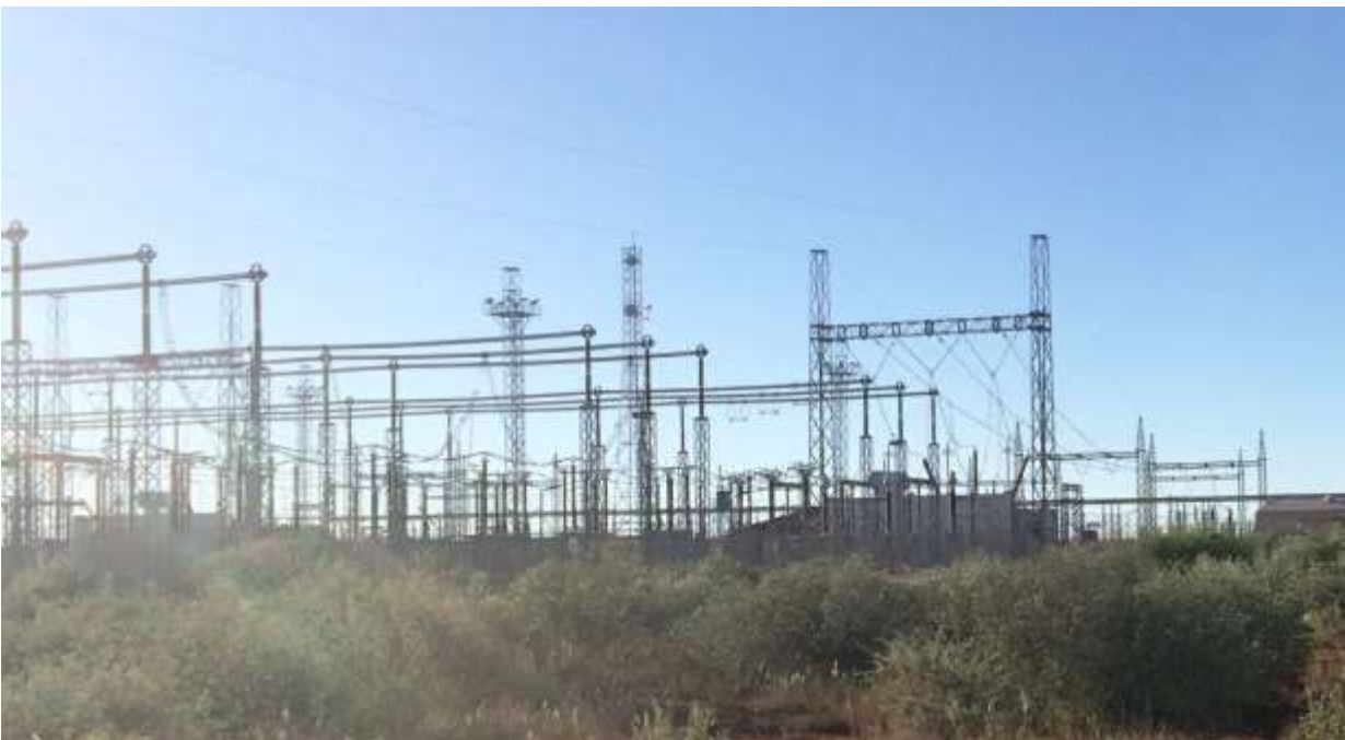
Figure 30: Photograph of the existing Eskom Mookodi Substation
