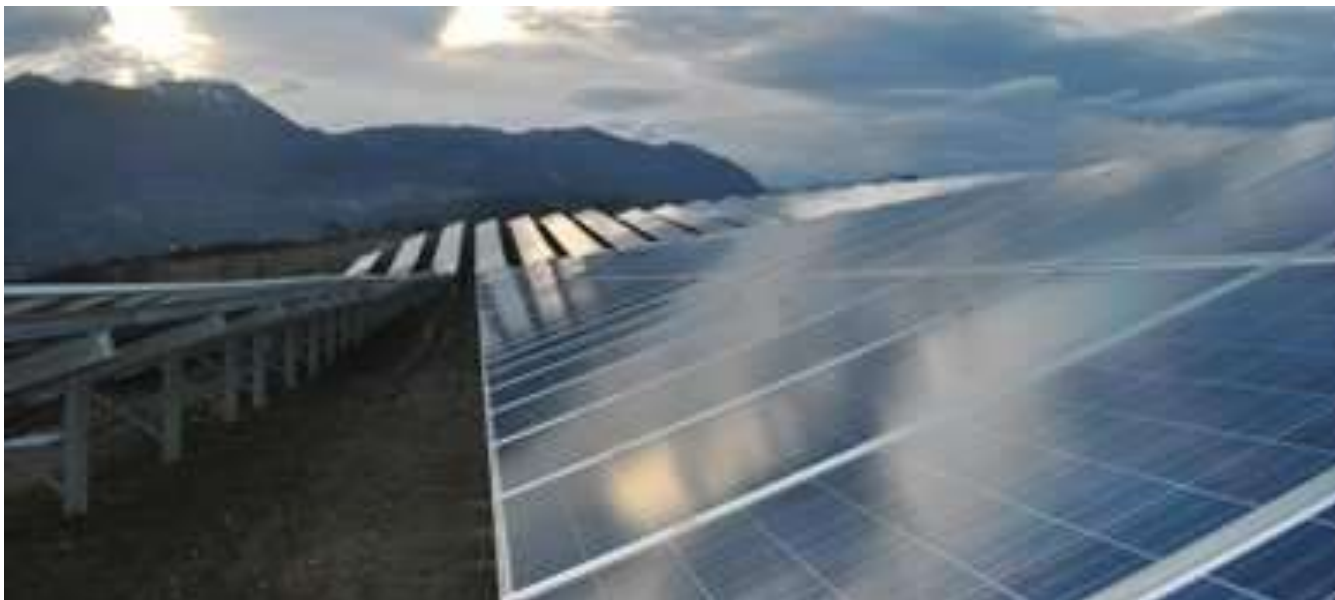
Figure 6: Examples of Fixed Rack Structures
