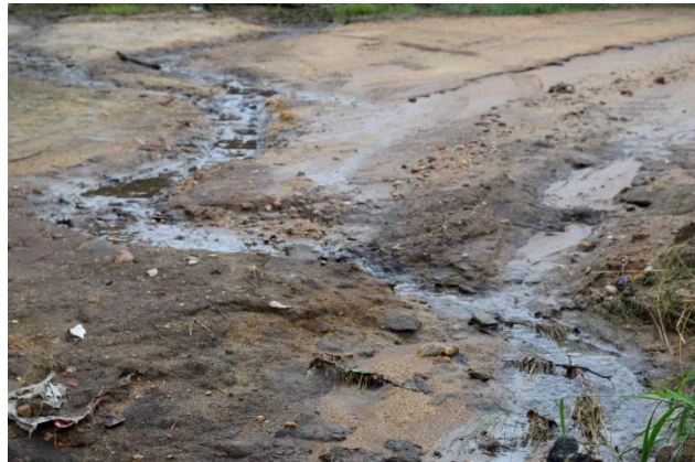
Soil erosion on the project site.
