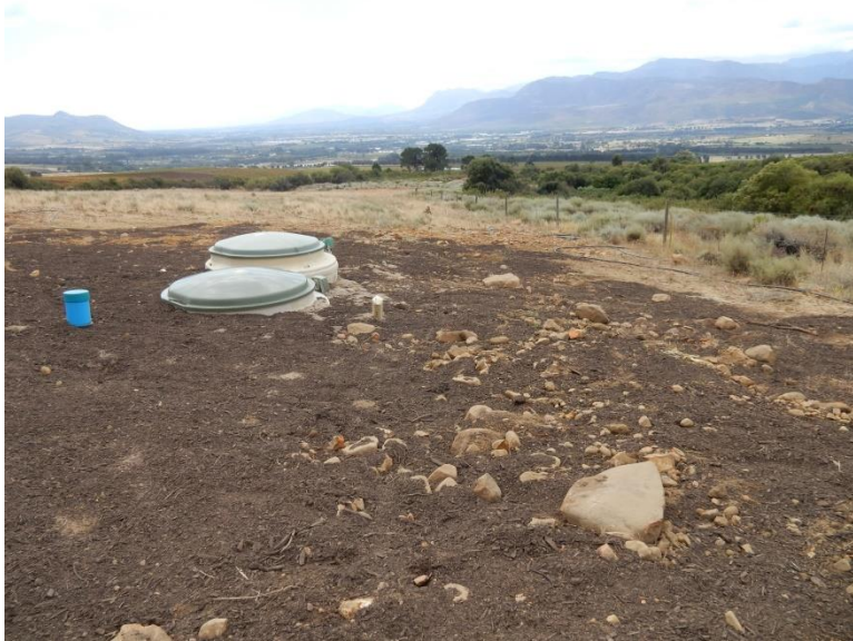
Figure 7.3 Above ground component of the BioDisc domestic sewage treatment plant (BA model), located at the Tented Camp site.
