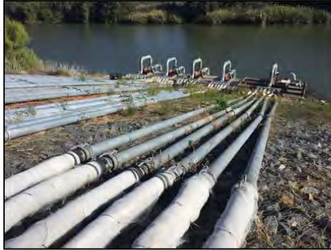
Figure 10: Existing pump station
