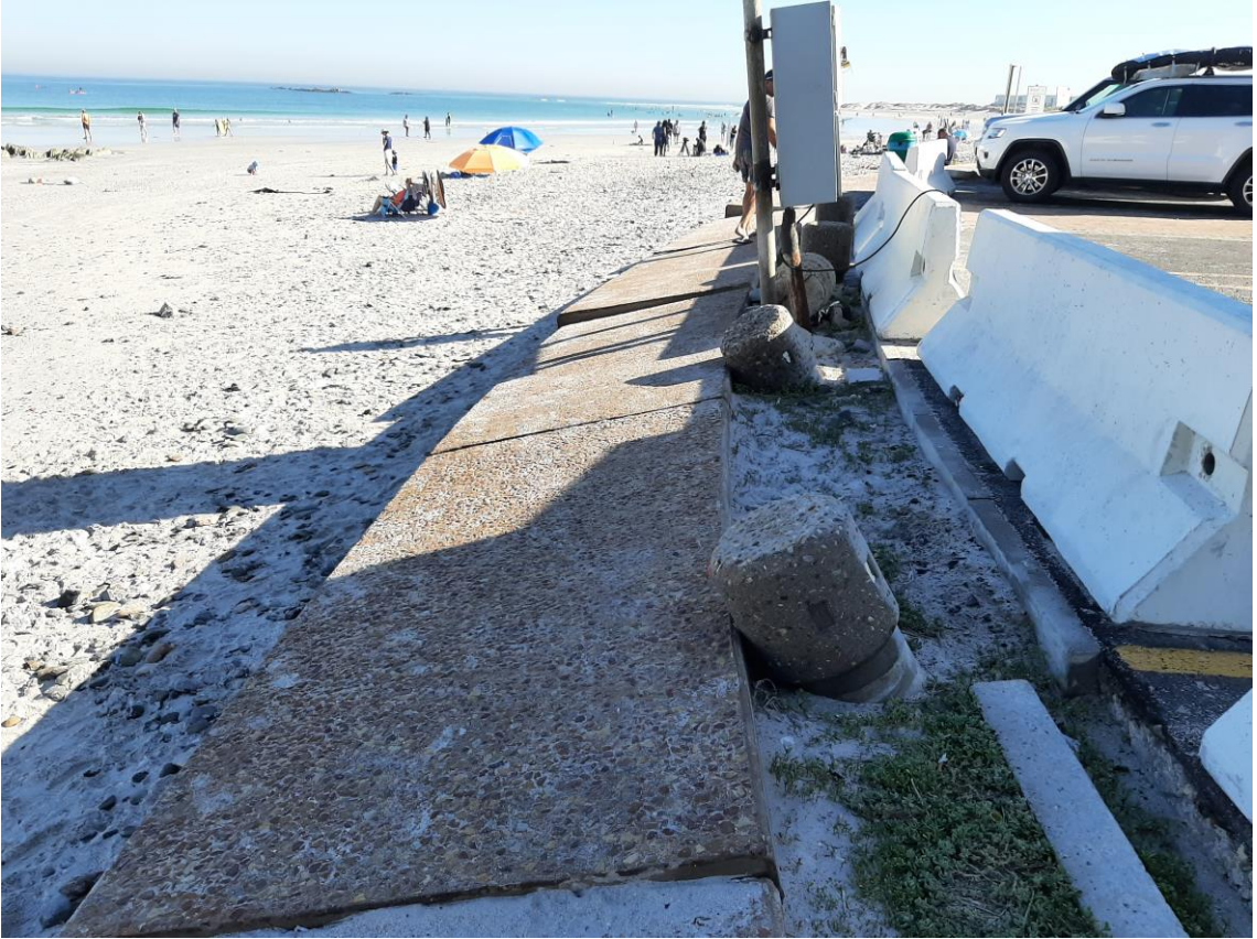
Figure 2.3: Settlement of seawall and sidewalk along De Mist public parking
