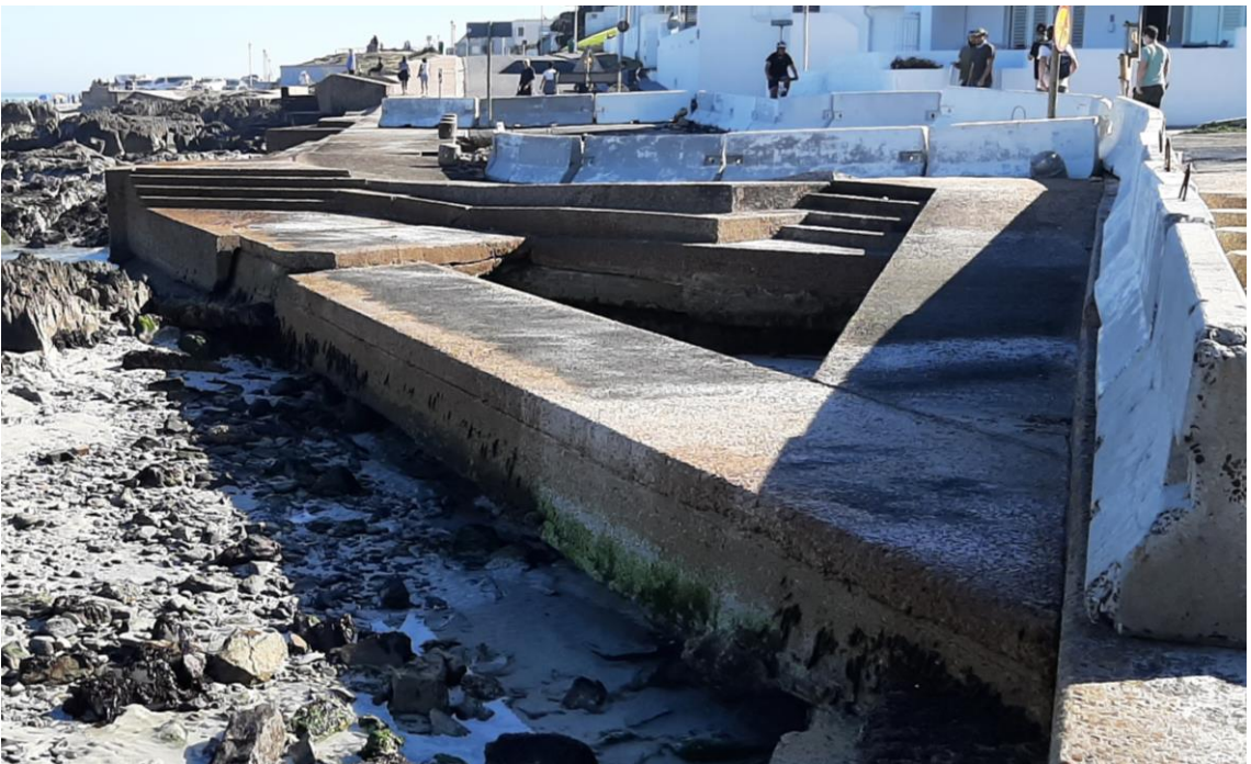
Figure 2.4: Undermined seawall along Popham Street
