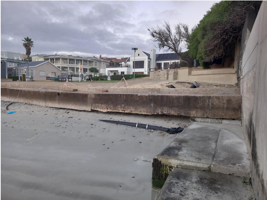
Figure 2.9: Undermining at Play Park showing cavity beneath the seawall and damage behind it.
