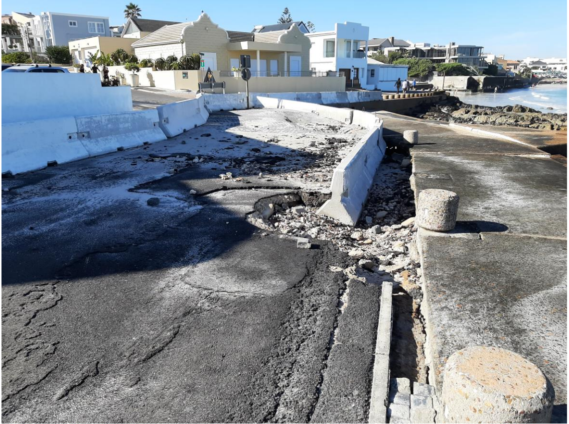
Figure 2.5: Popham Street structural failure
