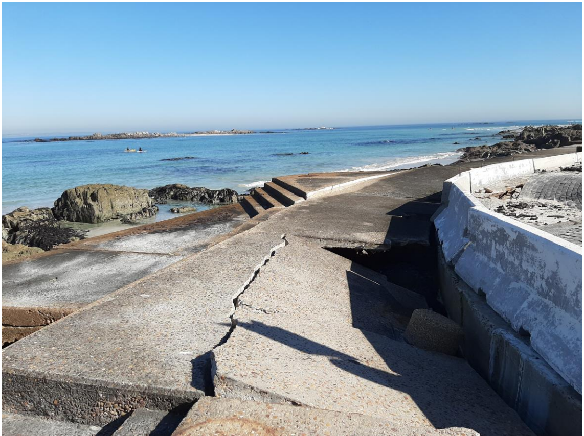
Figure 2.6: Popham Street sidewalk collapse
