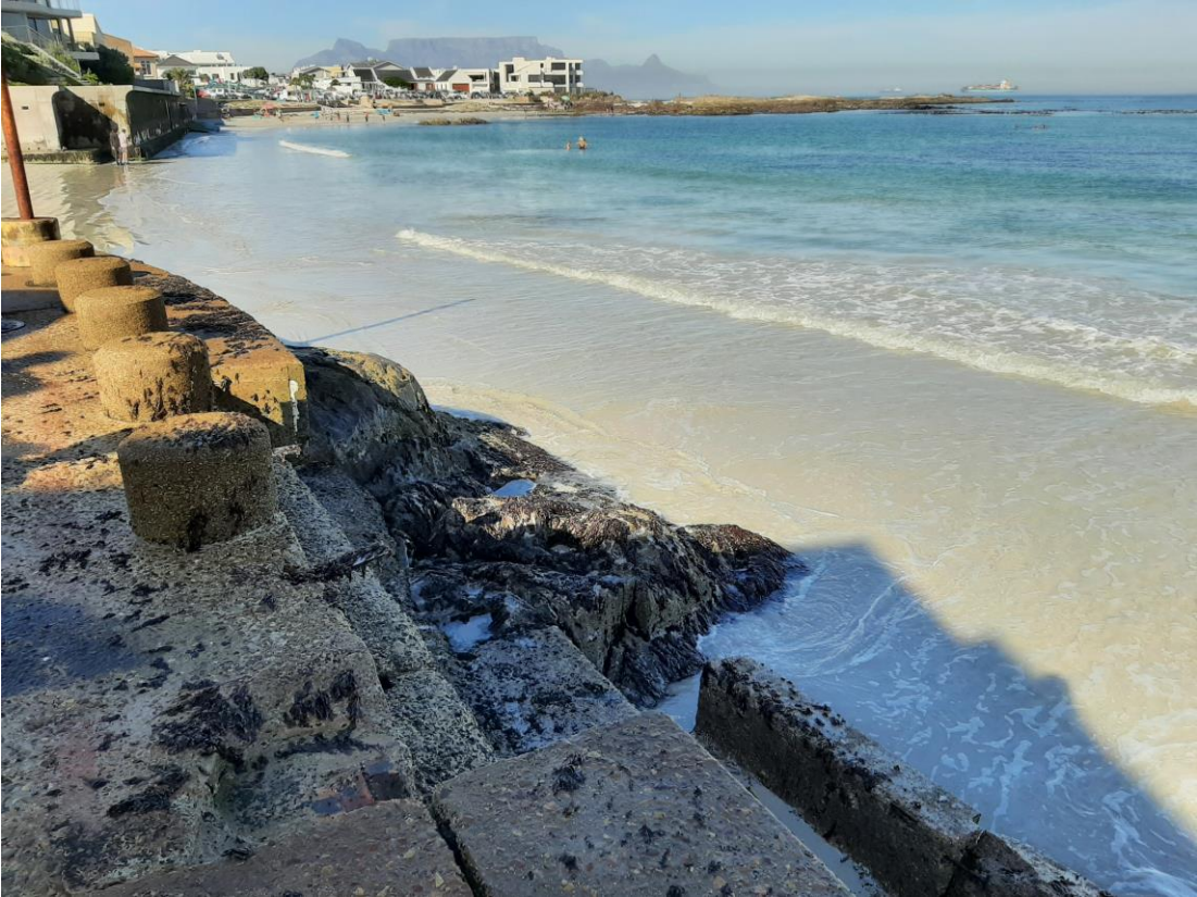
Figure 2.8: Localised failure of seawall along Pelegrini Street
