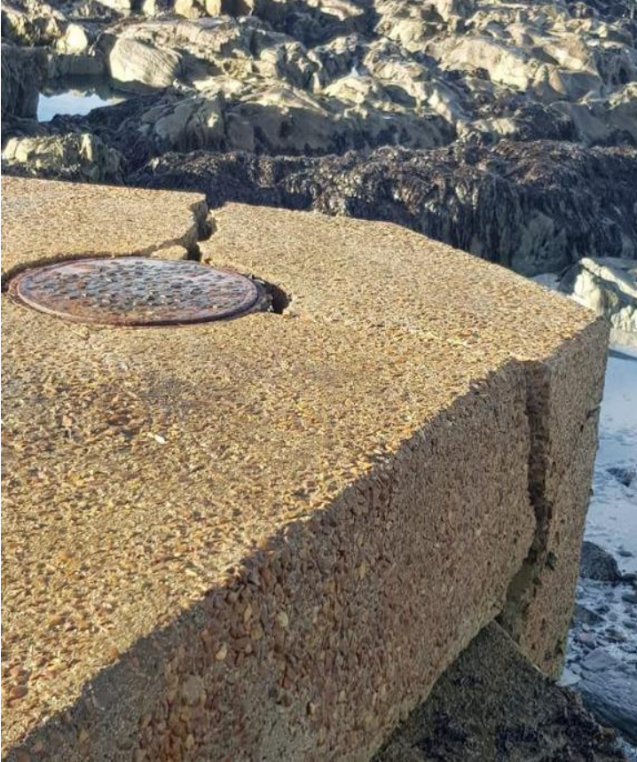
Figure 2.7: Sewer manhole breaking away from seawall.
