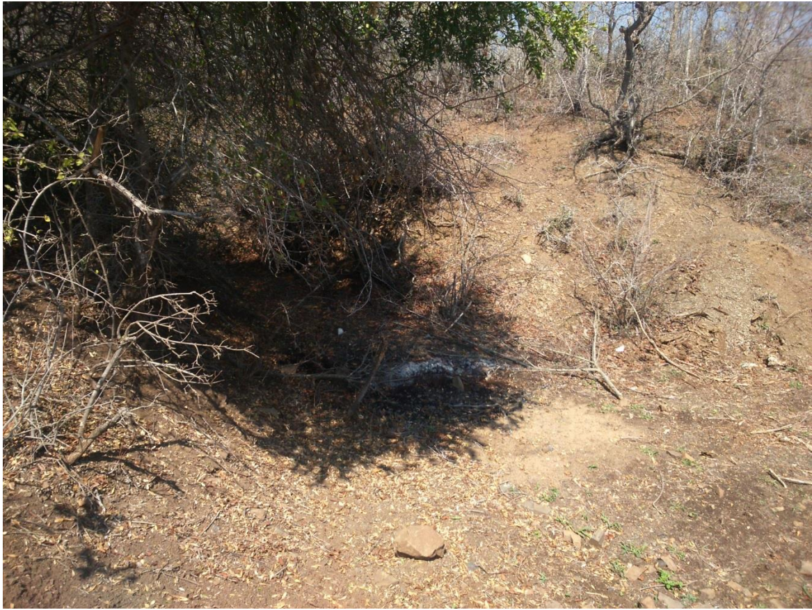
Figure 5: Image showing one of the pipe crossing areas which is seasonally wet.
