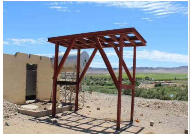
Photo 4: Contractors generator building, fuel storage
