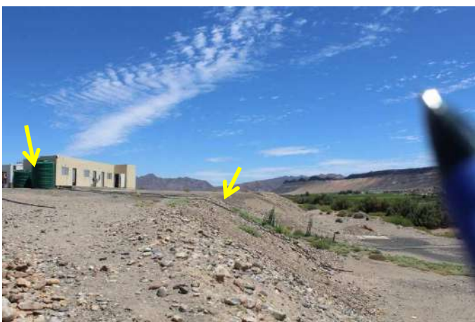
Photo 5: Water supply (JoJo tanks) and pipeline to Orange River abstraction point at contractors area
