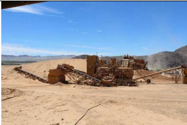
Photo 9: Standard Rotary Pan Plant (2 x 14ft) with ramp behind. This plant will be retained for mining phase.
