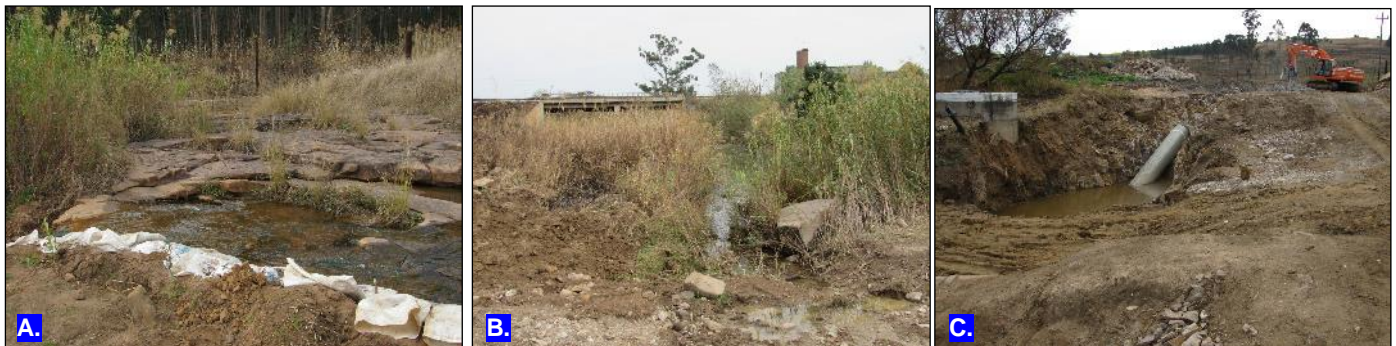
(a): Upstream of WC1 (b): Downstream of WC1 (c): Umgeni Water bulk pipeline currently under construction across the Mhlalane River during the time of the site inspection in August 2016.
